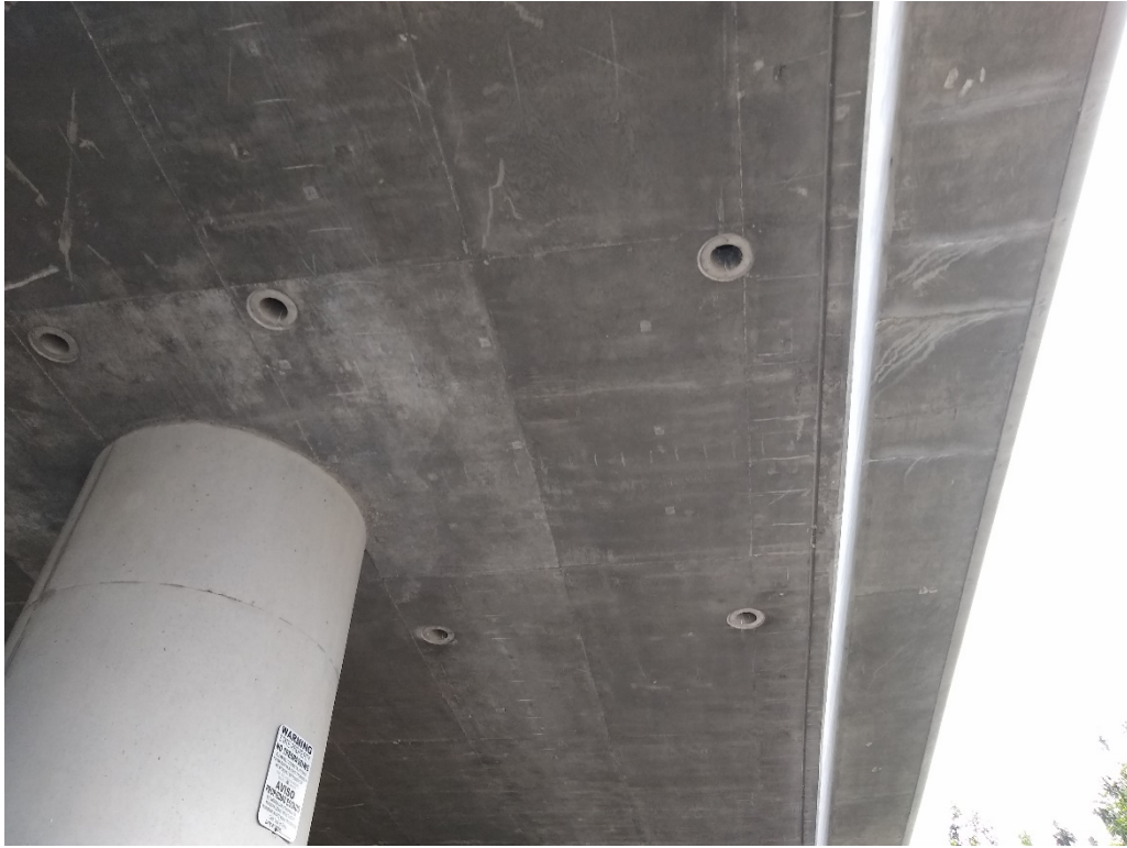
Photograph 9 – Firestone Boulevard under the I-605 bridge, bird droppings in holes.
